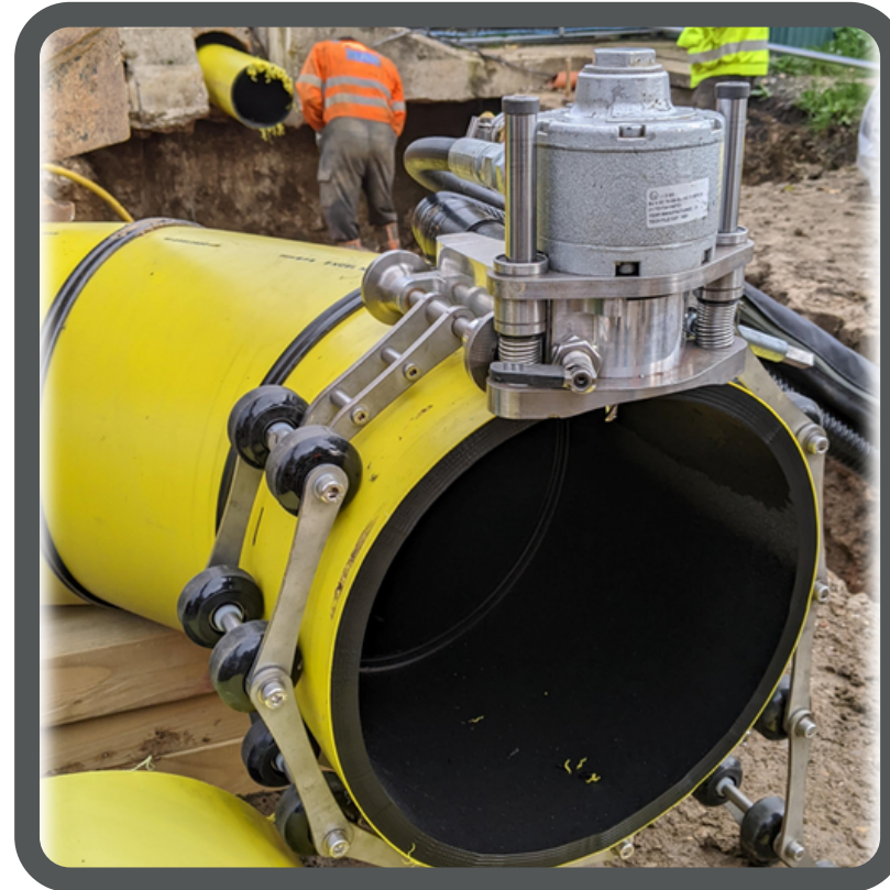
The PE Pipe Cutter on field trial at a site in Chelmsford. This pipe was 400mm and cut in just over two minutes.
