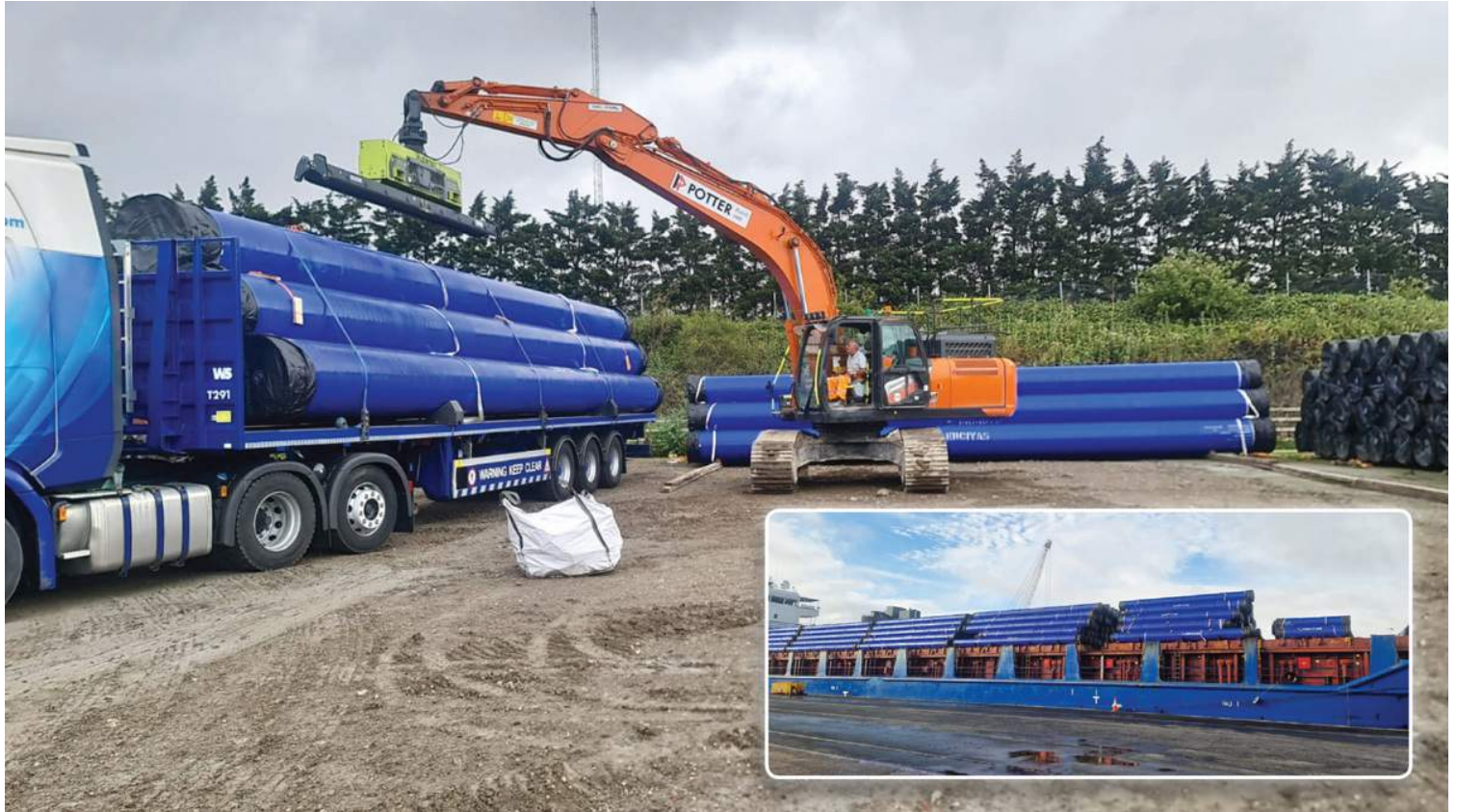
Figure 9: Delivery of steel pipes to the site and (inset) pipes arriving in the UK (courtesy of FT Pipeline Systems)
