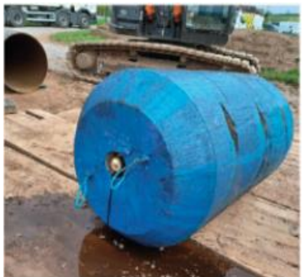
Figure 4 - A camera PIG was used to CCTV the main post cleaning.
