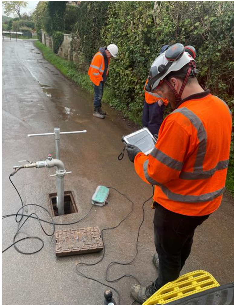
Monitoring location showing GPS system, Toughbook and Pressure Transducer.
